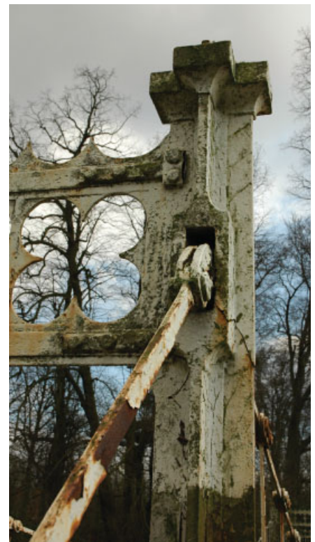
Fig. 8. Cast iron column with corrosion crack (2007)
