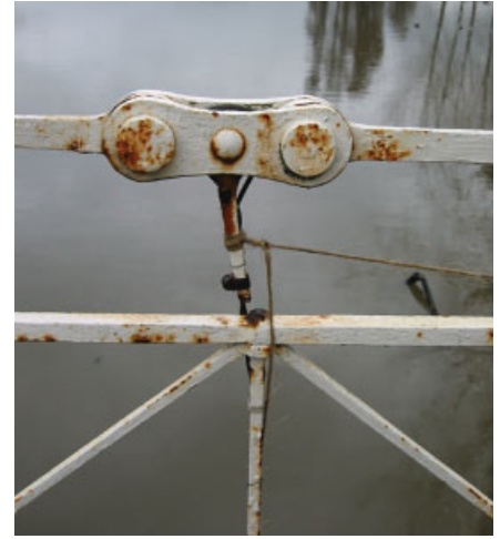
Fig. 7. Due to torsion of the bridge deck and corrosion, the vertical hanger has broken. The central bolt is not original (2003)
